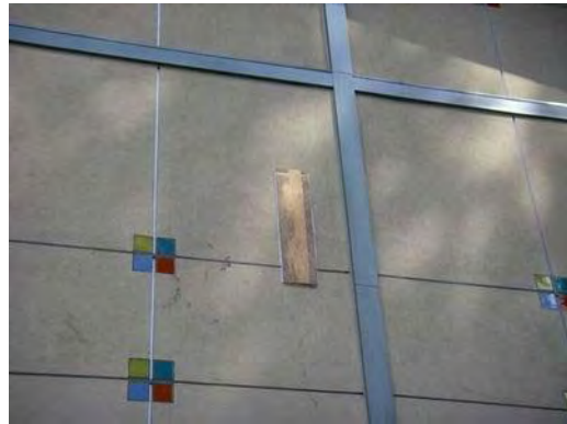
WALL DAMAGED FROM FALLEN TREE
