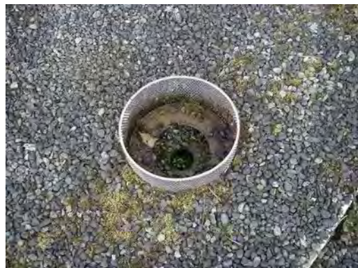
MISSING ROOF DRAIN SCREEN
