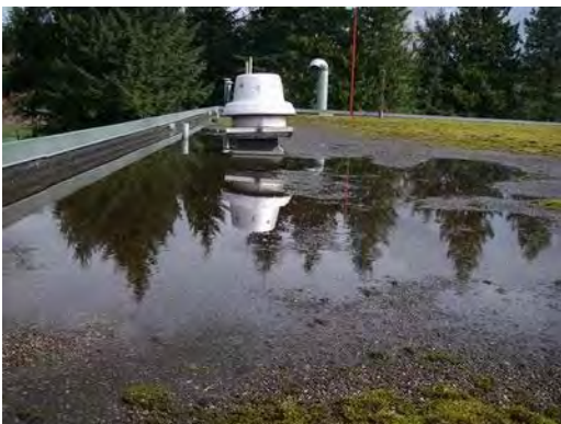
PONDING WATER ON ROOF
