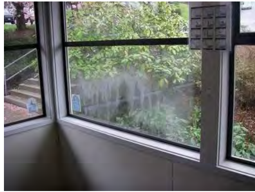
FAILED WINDOW SEAL
