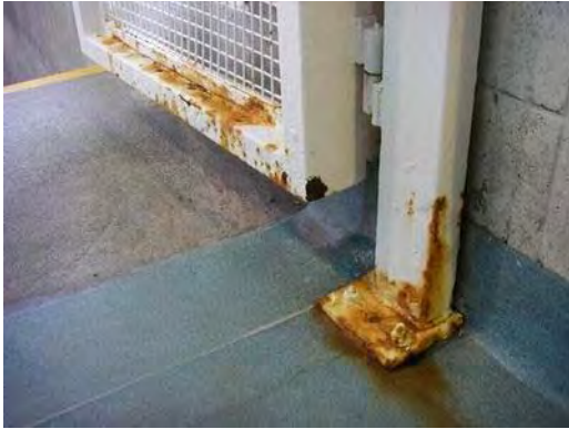
METAL GATE CORROSION
