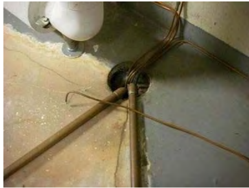
LEAKING FLOOR DRAIN
