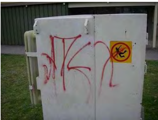
GRAFFITI ON TRANSFORMER
