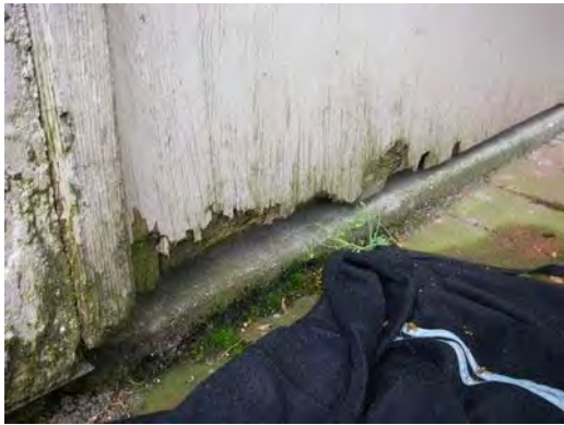
WATER DAMAGE TO DOOR
