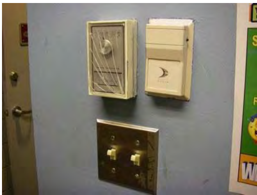
DAMAGED THERMOSTAT CONTROLS
