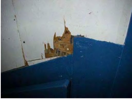
HOLE IN WALL
