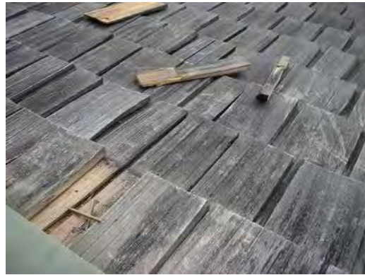
DAMAGED WOOD SHINGLE ROOF
