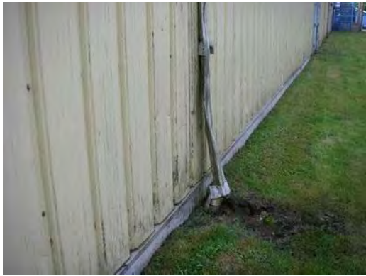
ROOF DOWNSPOUT DENTED
