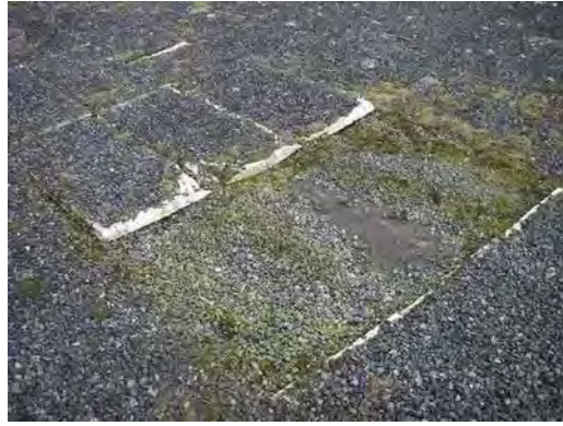
DISPLACED ROOF INSULATION
