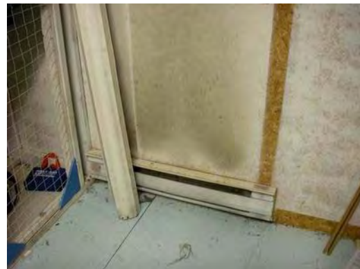
BASEBOARD WALLS STAINS
