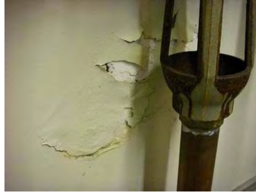
LEAKAGE INTO SPRINKLER ROOM
