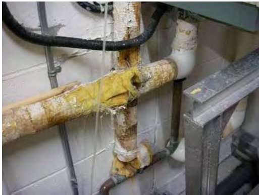
DAMAGED PIPE INSULATION
