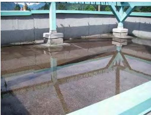
PONDING WATER ON CANOPY
