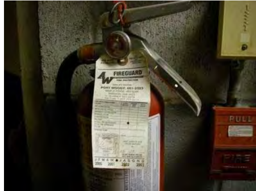
OUTDATED EXTINGUISHER TAG
