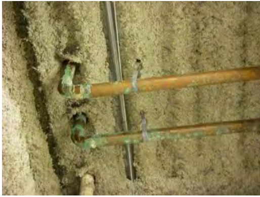
ELECTROLYSIS OF COPPER PIPING
