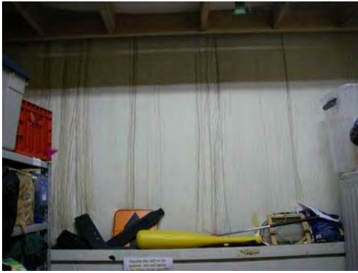
WATER RUNDOWN STAINS
