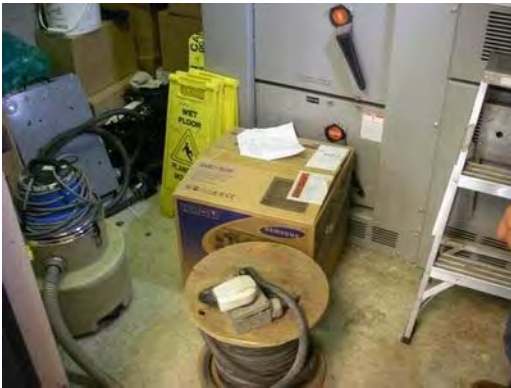
STORAGE IN ELECTRICAL ROOM
