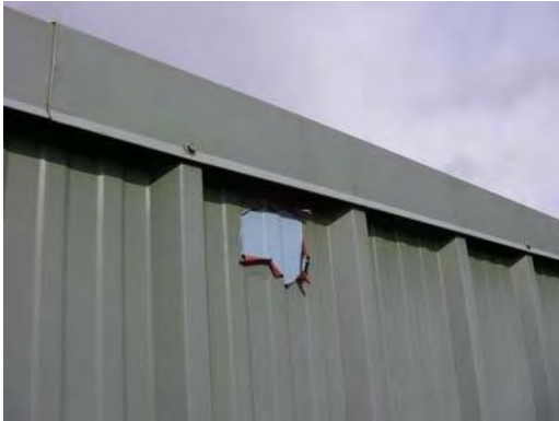
COATING PEELING ON METAL WALL
