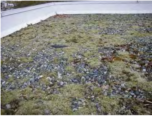
MOSS GROWTH ON ROOF
