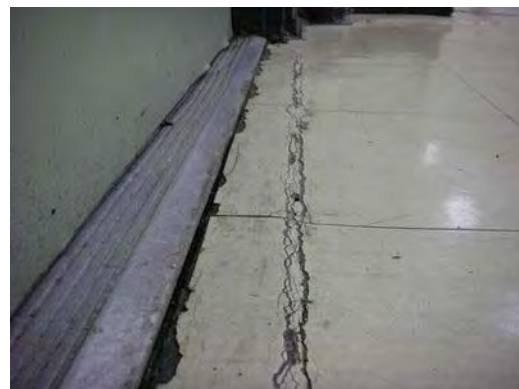
CRACKED RESILIENT FLOOR
