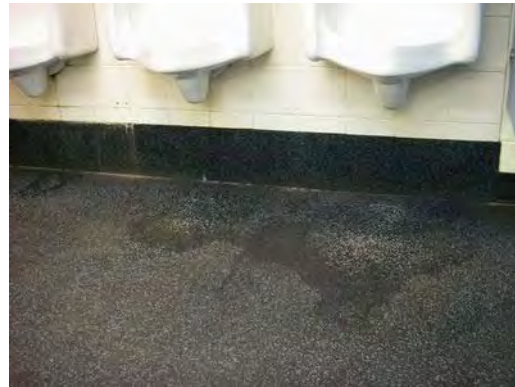
URINE STAINS ON FLOOR
