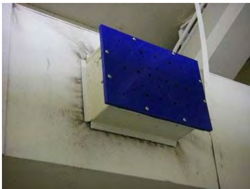
VENTILATION DIRT STAINS
