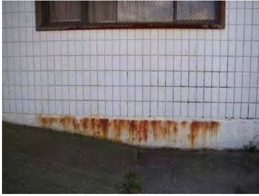
CORROSION STAINS FROM WINDOW
