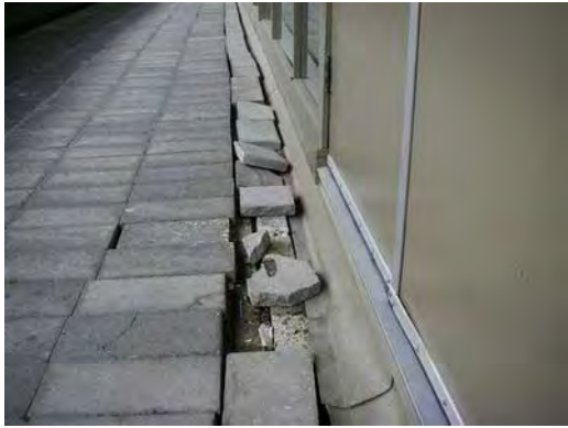
DAMAGED DECK PAVERS
