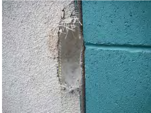
DAMAGED EIFS WALL
