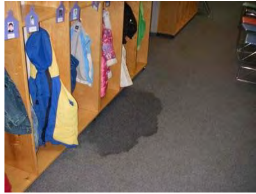
WATER STAINED CARPET
