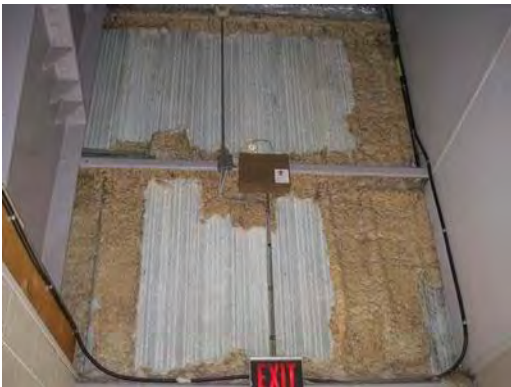
WALL INSULATION MISSING
