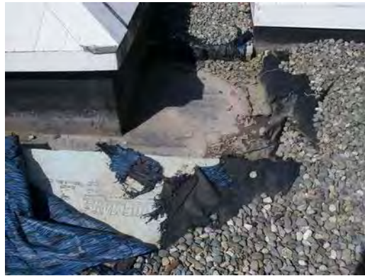
ROOF MEMBRANE EXPOSED
