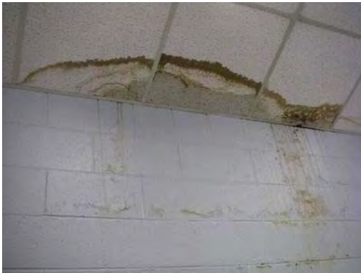
WATER STAINED CEILING TILE
