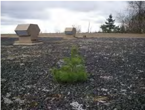
VEGETATION GROWTH ON ROOF
