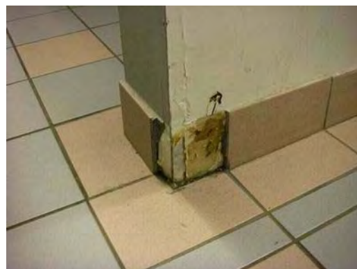
DELAMINATED FLOOR TILE
