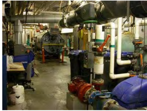
POOL MECHANICAL ROOM
