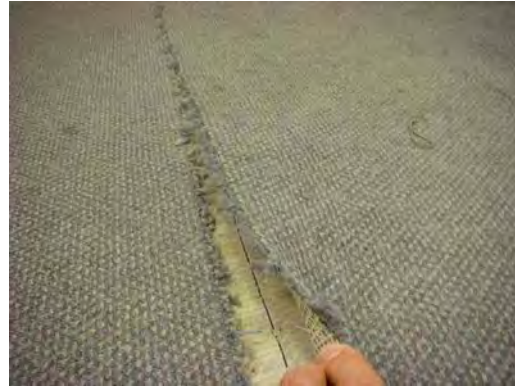
RIPPED CARPET SEAM
