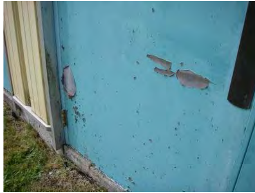
PAINT SCRATCHES ON DOOR
