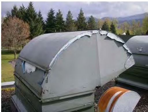
PAINTE PEELING ON HOUSINGS
