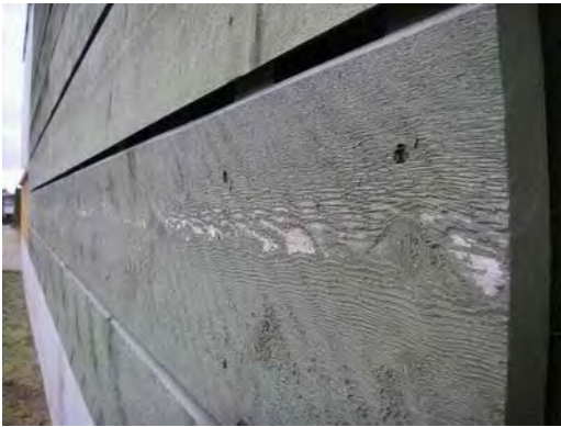
DAMAGED WOOD FASCIA
