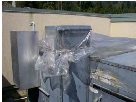
PLASTIC ON AHU
