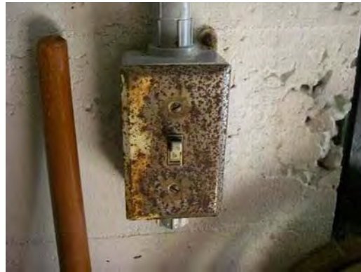
CORRODED LIGHT SWITCH
