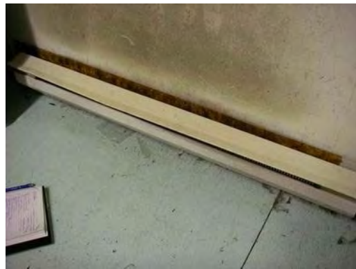
LOOSE BASEBOARD HEATER
