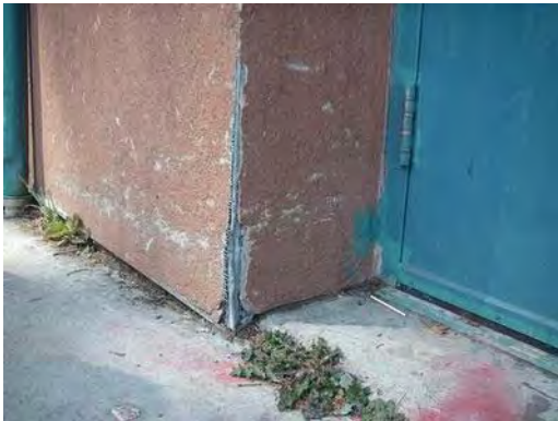
DAMAGED STUCCO WALL
