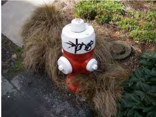
GRAFFITI IN FIRE HYDRANT
