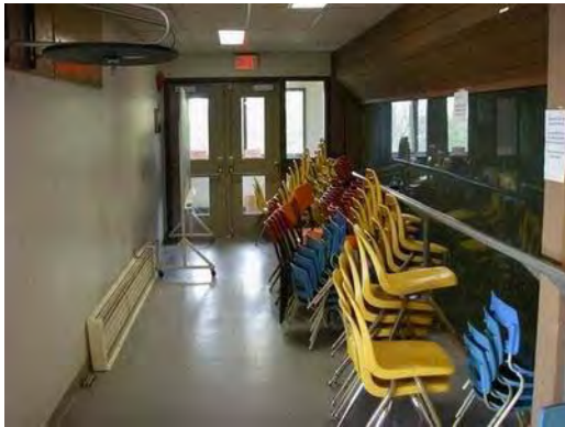
BLOCKAGE IN FGRESS ROUTE
