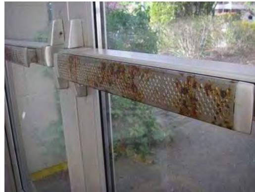
CORRODED DOOR PANIC HANDLE
