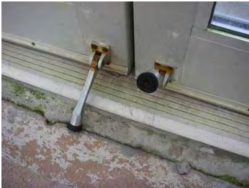
CORRODED DOOR STOP
