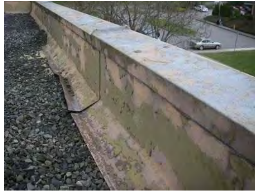
PAINT PEELING ON FLASHING
